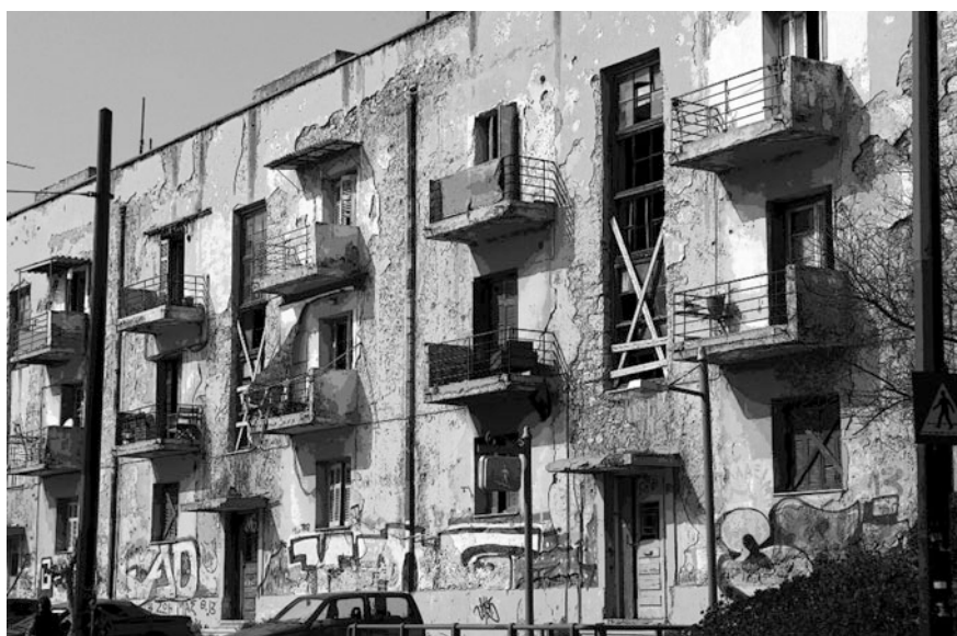
Fig. 4.2 View of the refugee housing estate on Alexandras Avenue, central Athens, 1933–1935. Source Maloutas, personal archive, 2009
